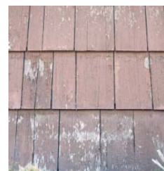
Painted over weathered wood. Improper installation.
