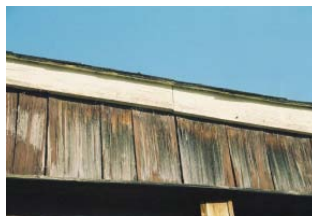
Not back primed. Weathered wood and mold
